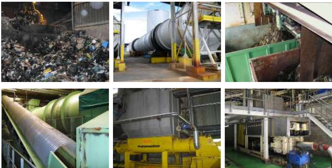
Figure 6. Dry digester material handling equipment.
